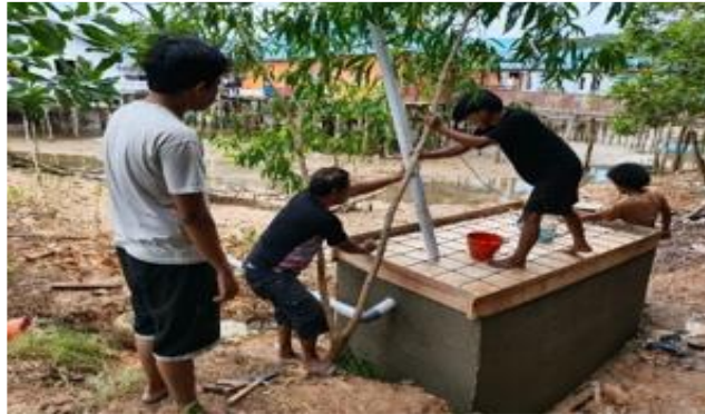
Figure 5. Construction Implementation, Such as Making Waterproof Walls and Floors, Installing Inlet-Outlet Pipes
